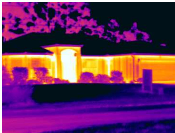
Description: IR Image #15 Thermal image of neighboring home with CBS construction showing considerably more heat loss
