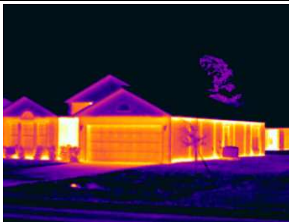
Description: IR Image #3 Thermal image of neighboring home with CBS construction showing considerably more heat loss
